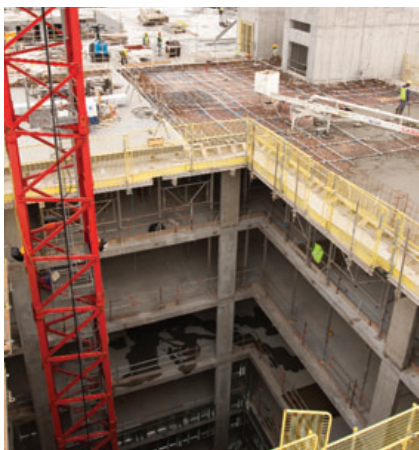
500 Lockable dowels were installed on the Emergency Care Centre in Aberdeen, UK
