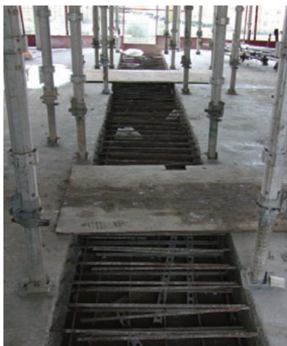
Pour Strips restrict site access, cause a trip hazard and delay progress on site
